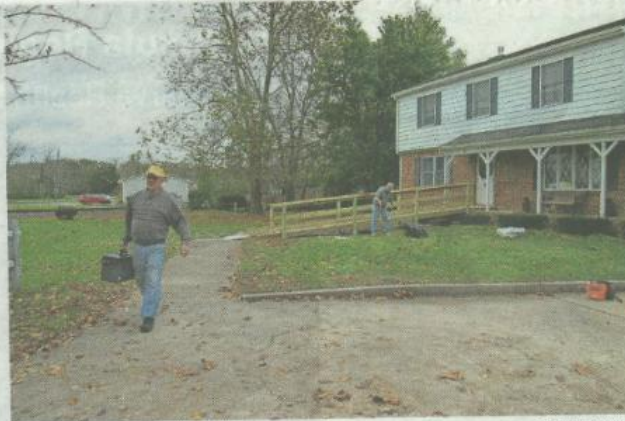
Members of the Lord Baltimore Lions Club build a wheelchair-accessible ramp at a Frankford home.
